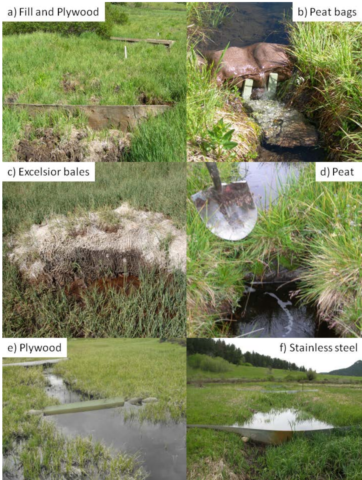
Figure 1. Examples of ditch filling and plugging techniques used in the Rocky Mountains, USA.
