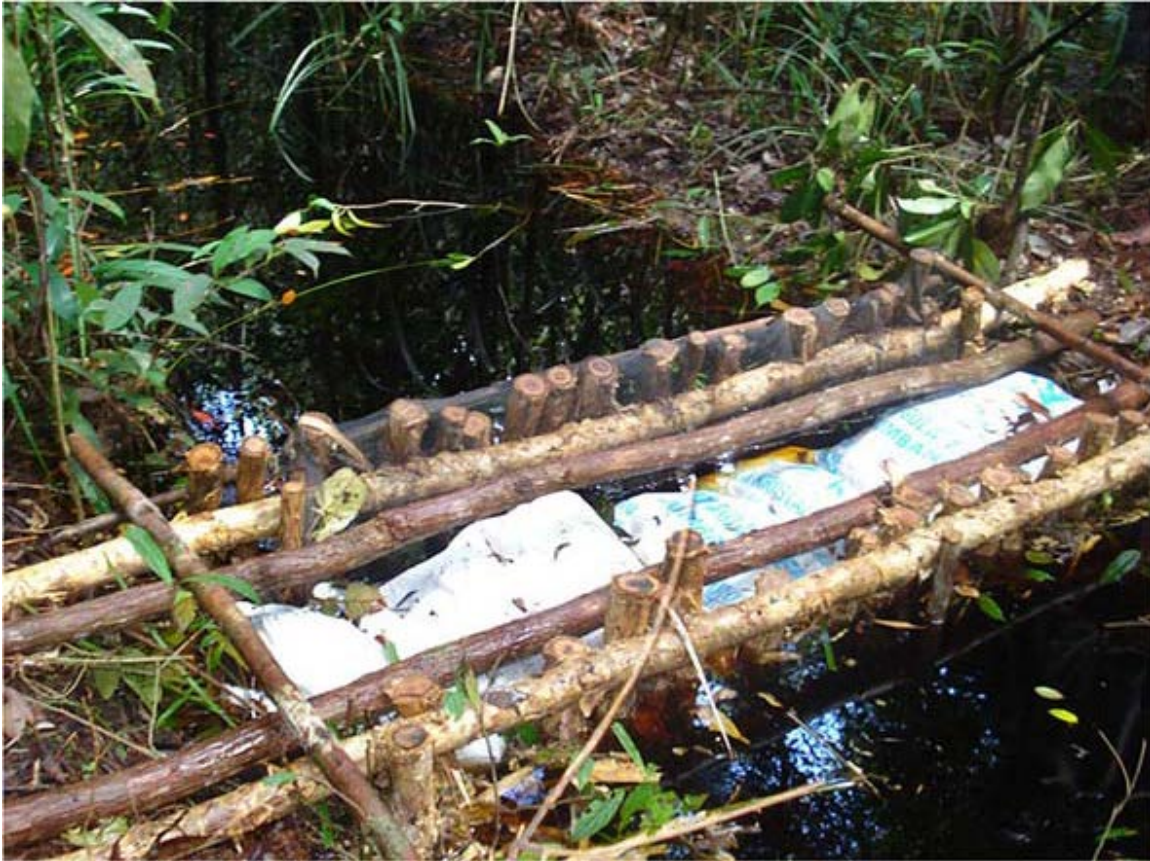
Fig. 3 Simple dam in the Bangah catchment made of locally available material (3 m long, 1 m wide and 2.5 m deep).
