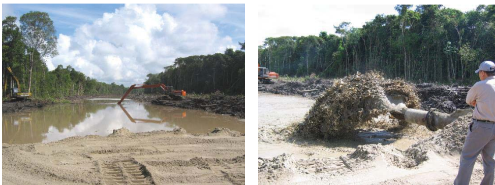
Figure 3. (a) (left) Fibrous peat excavation using long-arm excavators and (b) (right) Hydraulic sand-filling works in progress.
