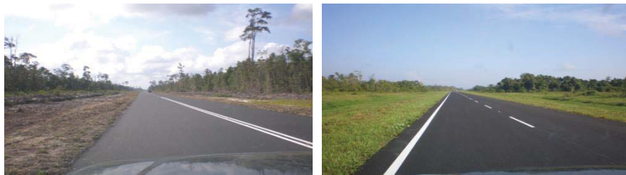
Figure 4: (a) (left) Just completed road and (b) (right) successful turfing of road shoulders.
