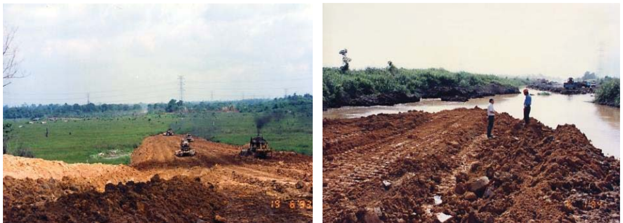
Fig. 2.1a & 2.1b : “Displacement Method” of Road Construction on Peat & Organic Soils along New Sibu Airport Road.
