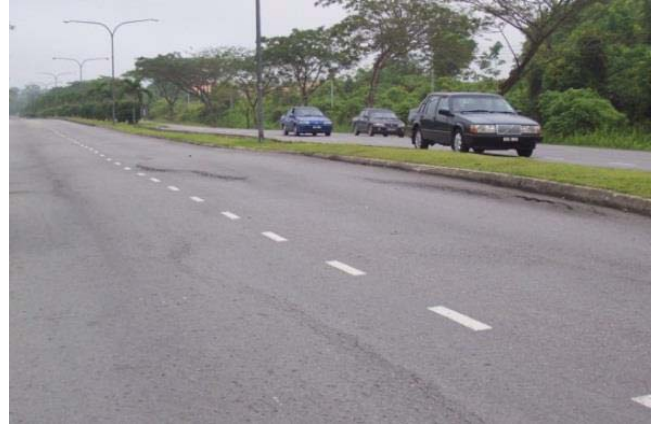
Fig. 2.1d : Highlight on the defects of Conventional Method of Road Construction on Peat & Organic Soils
