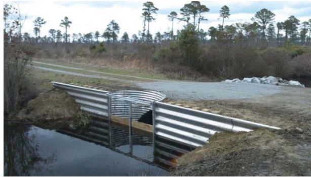
Figure 3: Recently installed water control structure at Great Dismal Swamp NWR.
