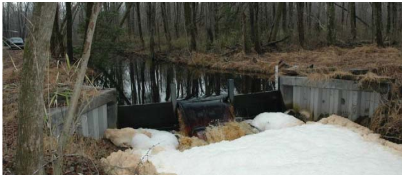
Figure 4: Example of an adjustable weir type water control structure. Weir width approximately 4.5 m. Great Dismal Swamp NWR. Photo courtesy David Byrd, USFWS.
